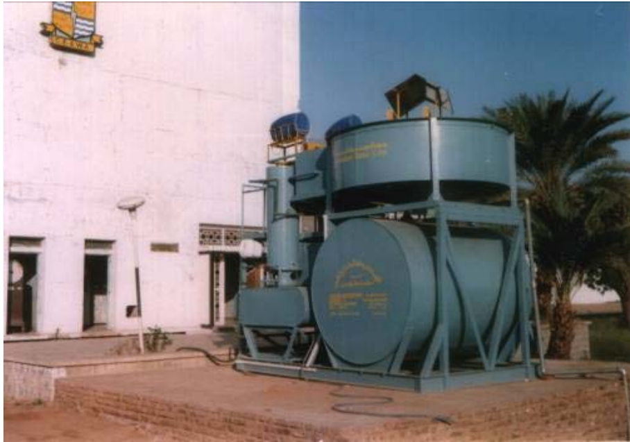
Photo D1 Khartoum Municipal Water Works – 1999 Mini Water Station For the Sudanese Standards and Metrology Organization
