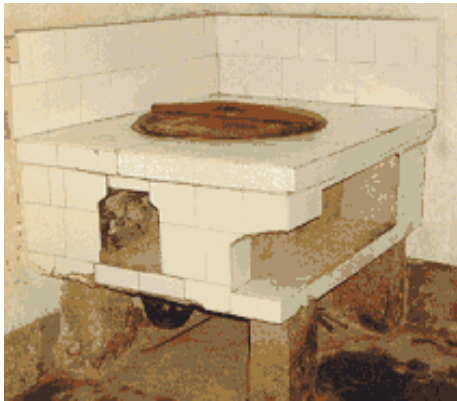
a) General appearance of the stove after installation with the (rear) chimney hidden by the wall. The cooking cauldron sits tightly over the combustion chamber and a space is provided for the air blower and the firing port
